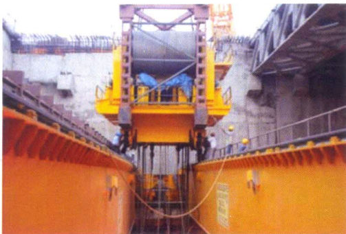
Figure 6. Trolley assembly being placed with the hooks on the bridge girder rails.
