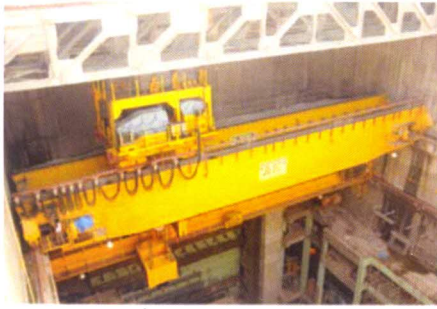
Figure 1. Overview of 280/85T EOT Crane in RCB.
